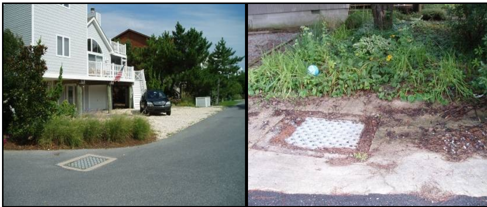
Figure 5. Examples of storm drain inlets that are not stenciled or marked. Left – N3 (South Bethany) and Right – N4 (South Bethany).
