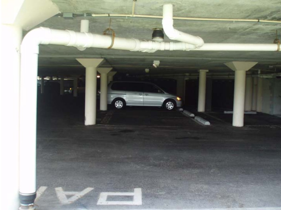
Figure 2: Drainage pipes collecting runoff from the promenade
