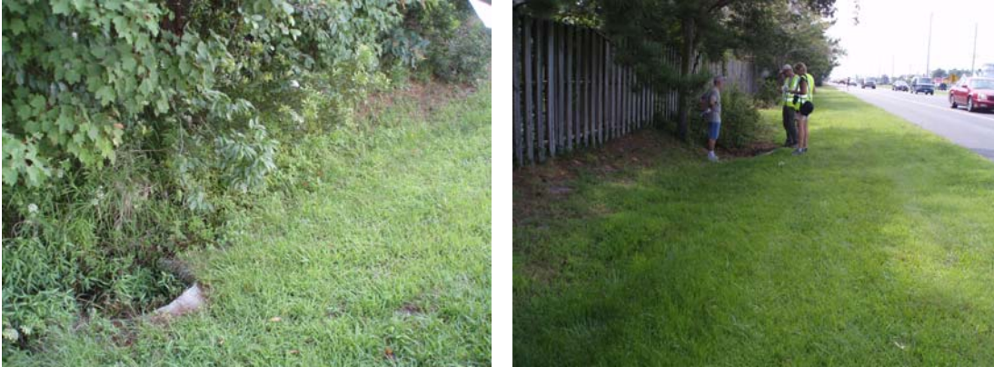
Figure 2: East side of Coastal Highway. Left: Partially filled stormwater inlet in Site R8. Right: Stormwater inlet and shallow swale in Site R5.
