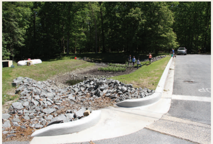
The reconstructed riprap inflow channel allows water to run into the area without eroding the hillslope
