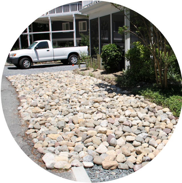
Image: Rocks covering the infiltration trenches were chosen to blend attractively with existing driveways and garden areas.
