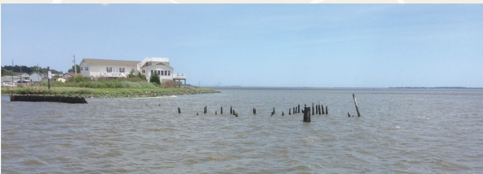
Partially submerged pilings at the entrance to the channel prior to the start of the project.
