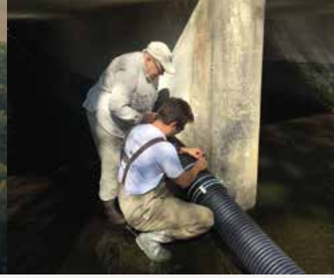
Board Chair, Susie Ball, and Environmental Scientist, Andrew McGowan, affix the eelway to a piling of the dam
