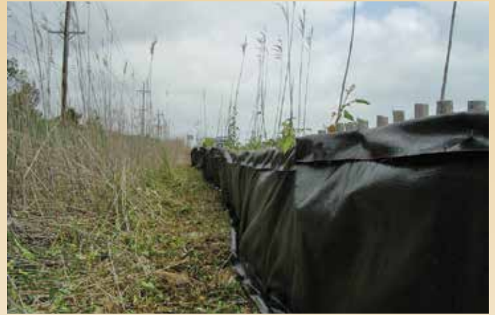
Diamondback terrapin fence with attached silt fabric Photo courtesy of Delaware Seashore State Park
